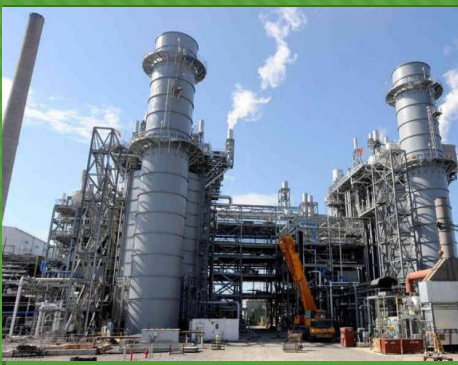
Sindh Nooriabad Gas Power Plant
